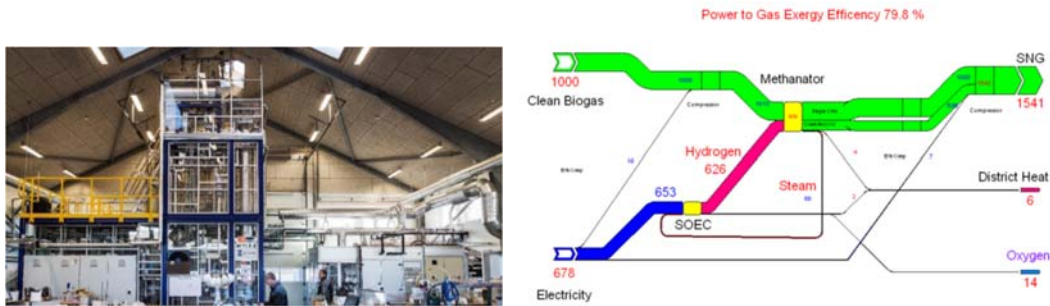
Figure 56 141 . Left: Haldor Topsøe biogas upgrading plant in Foulum, Denmark. The plant includes a 50 kW hydrogen-producing SOEC unit for steam electrolysis and catalytic methanisation, where CO 2 in the biogas is upgraded to pure methane of pipeline quality. Right: Exergy efficiency in the process is calculated to be approx. 80%.
