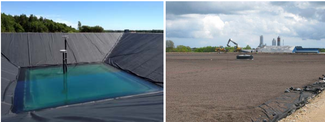
Figure 69. Left: Pit Thermal Energy Storage at Dronninglund in Denmark. The storage volume is being filled with water and the heavy plastic liner separating water from the soil is
