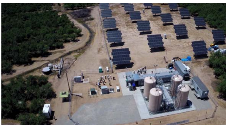
Figure 40. Photo of the EnerVault installation in California 100.
