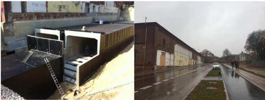
Figure 73 194 . Left: Construction of the cold storage facility. Left: Covering road after finishing.
