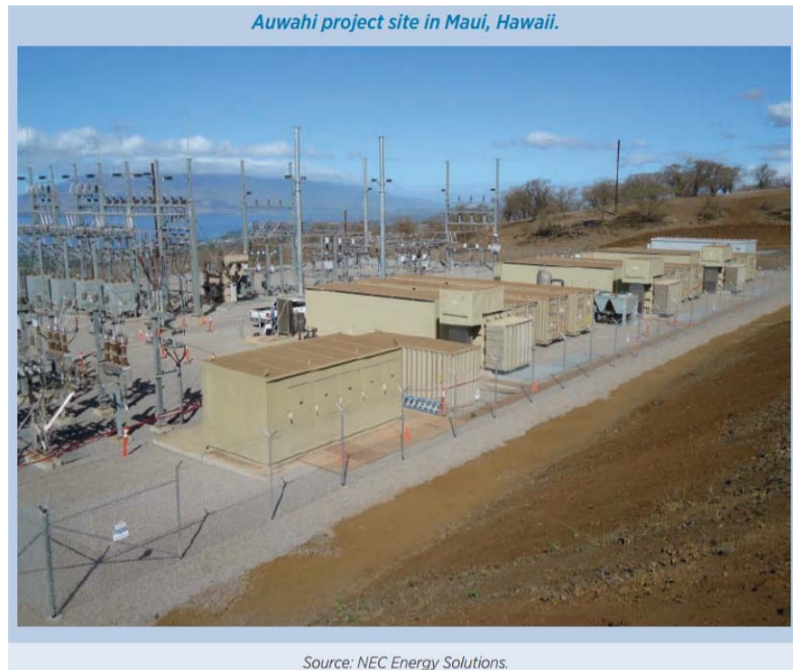
Figure 24. LIB based storage for onsite wind energy smoothing in Hawaii.
