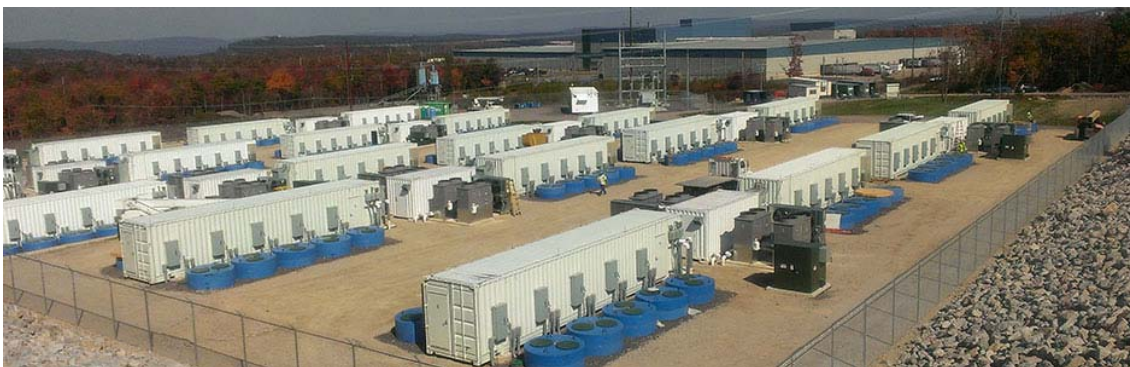
Figure 78. Photo of Beacon Power flywheel installation in commercial operation in PJM, Hazle, Pennsylvania. The plant includes 200 flywheel modules lowered into the ground (5 on
